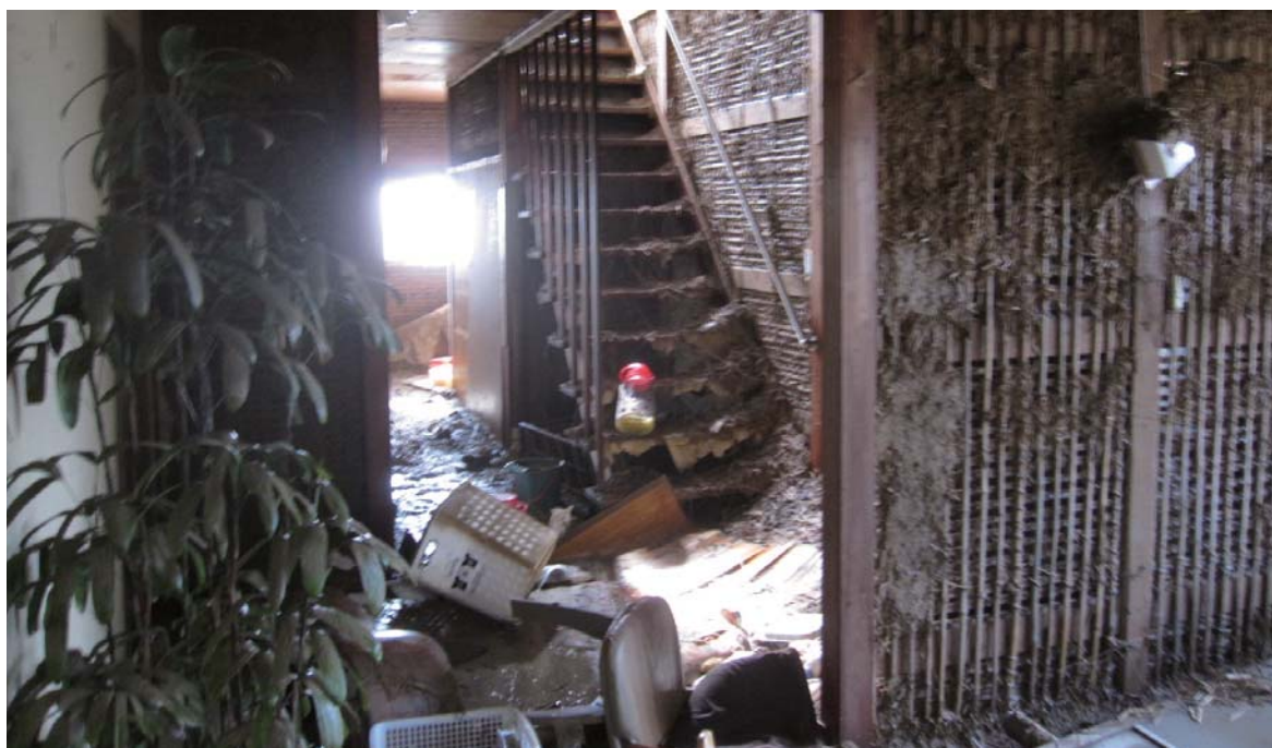
Inside a damaged building
