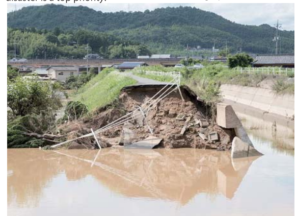
An embankment that collapsed due to a mud flow When the embankment broke, flooding of homes progressed quickly. Sediment inflow and damage to houses occur near the site of collapse.
